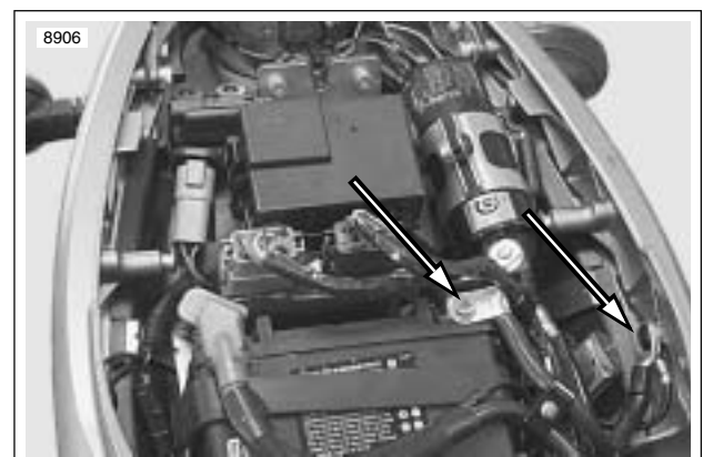
Figure 7-39. Negative Battery Cable
