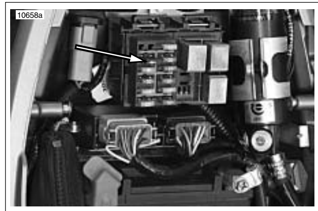
Figure 7-17. Fuse Block (contains diodes)
